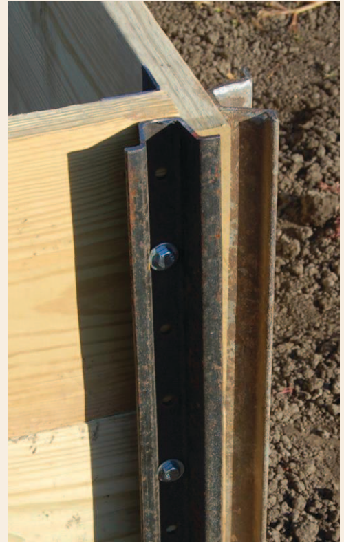
Figure 10. This GB in Morris, MN uses fence posts, lag screws, and angle irons in the corners.
